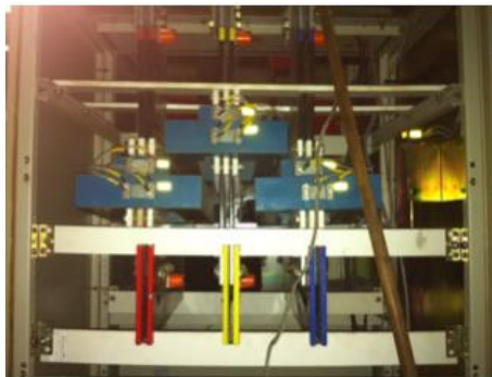
SM's installed on bus bars
